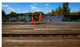
Network Rail workers in Sheffield repair and replace stolen copper wiring. Photographer: Christopher Thomond for the Guardian
